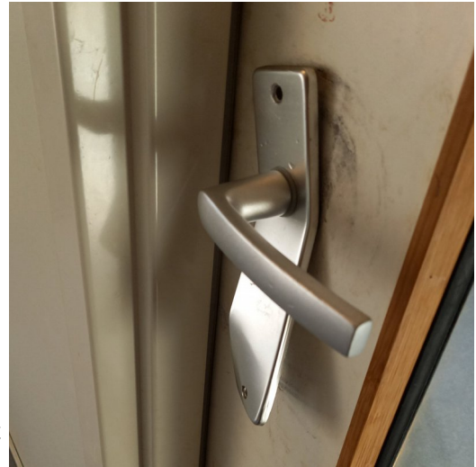
Door handle was damaged by the refugees. Likely during some fight.
